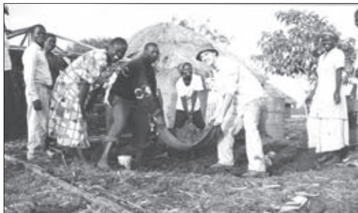
Tim's first project in Kenya consisted of helping to build three mud huts for the elderly. "I donated much of the flesh on my palms as I learned how to use a machete to cut timber". Tim is shown carrying soil towards the site of one of the huts.
